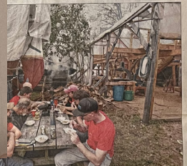
Steve Denette, left, and his crew take a break for lunch during a day of steaming, bending and installing frames for the Arabella, taking shape in the boatworks at right.
